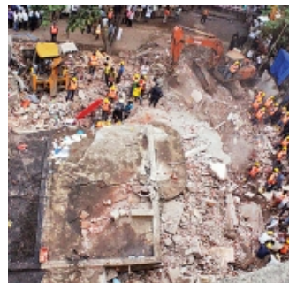
Thane: After fall of residential building, 480 schools 'sans OC' could be next
